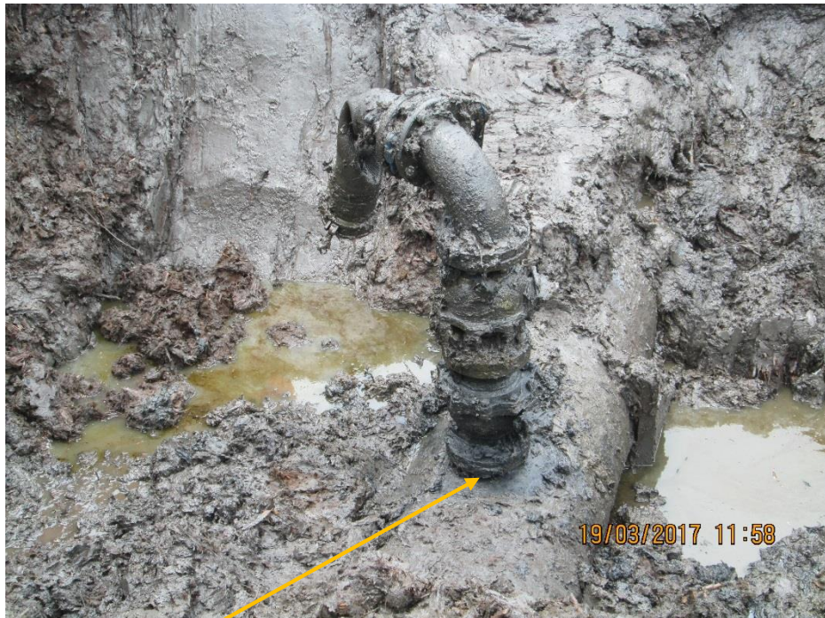
Close-up: Illegal fitting on 28" Bomu-Bonny Trans Niger Pipeline at Owokiri. Picture was taken during Joint Investigation of 19 th March 2017.
