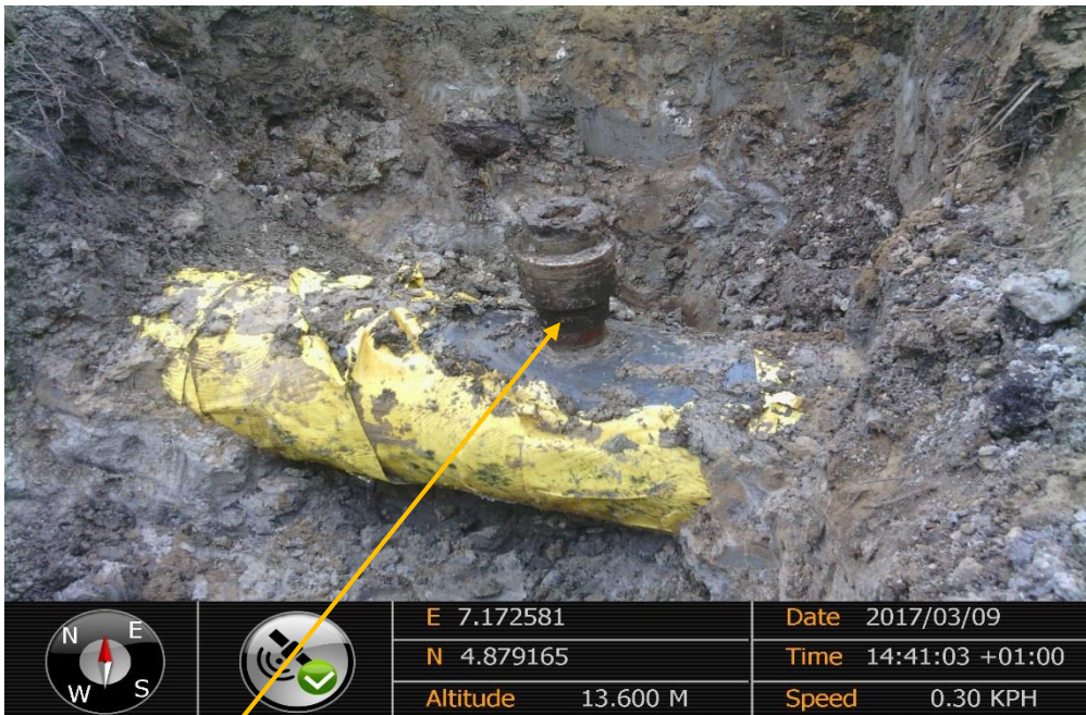
Close-up: Illegal fitting on 12" Imo River-Ogale Pipeline at Komkom. Picture was taken during Joint Investigation of 9 th March 2017.
