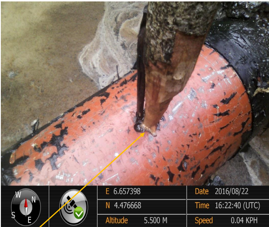
Close-up: Plugged drilled hole on 8"Belema-Sego Delivery line at Offoinama. Picture was taken during Joint Investigation of 22 nd August 2016.
