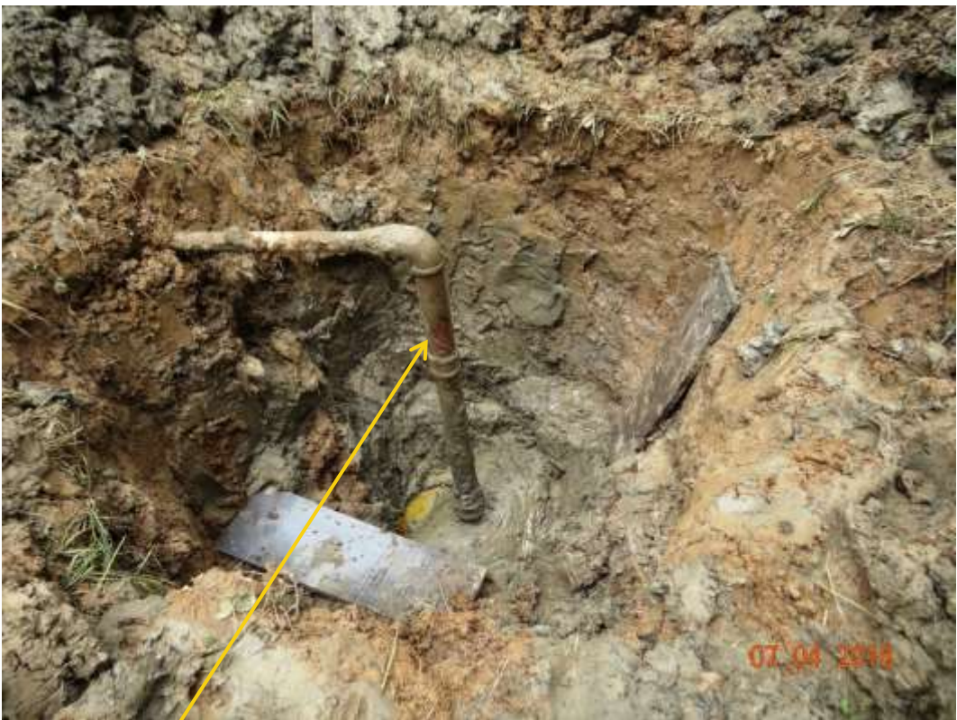
Close-up: Illegal fitting on 20" KoloCreek – Rumuekpe Trans Niger Pipeline at Odau. Picture was taken during Joint Investigation of 7 th April 2016.
