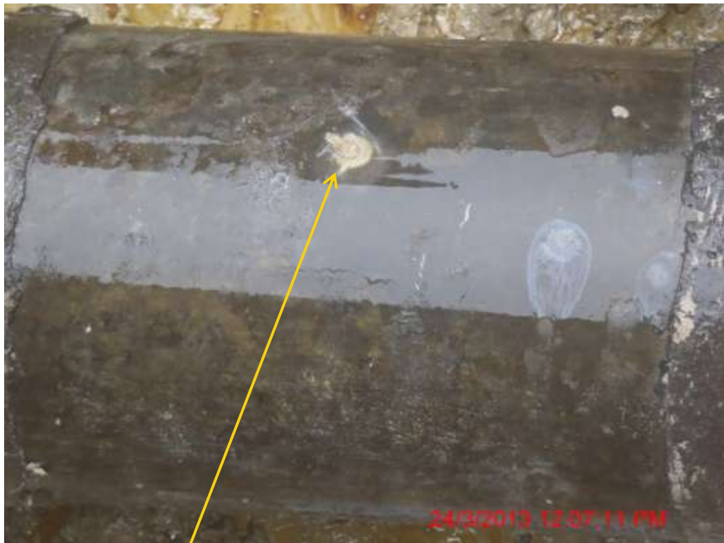
Close up: Drilled hole on 12" Oguta-Egbema pipeline at Obiakpu. Picture was taken during Joint Investigation of 24 th March 2013.
