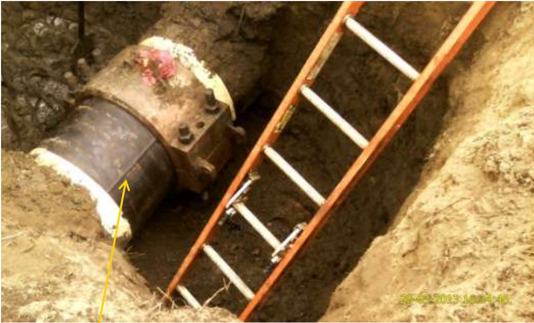
Close up : Former location of missing clamp on 24" Nkpoku-Bomu pipeline at Bera. Picture was taken during Joint Investigation of 28 th March 2013.
