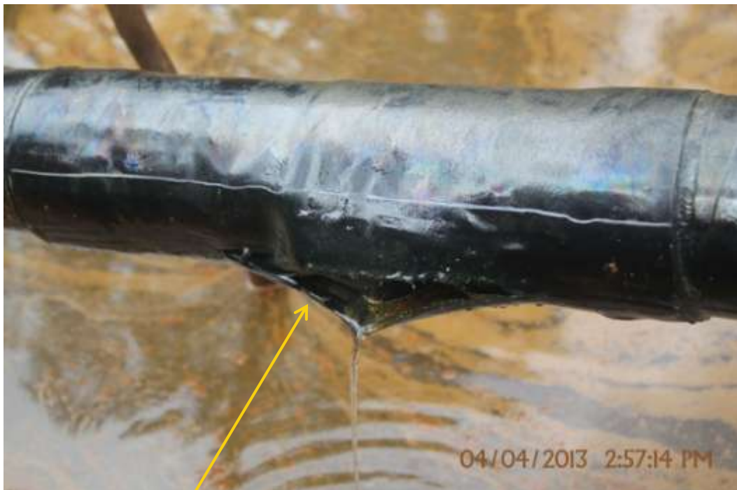
Close up: Raised pipe on Opukushi Well34T flowline at Egbemo-Angalabiri. Picture was taken during Joint Investigation of 4 th April 2013.
