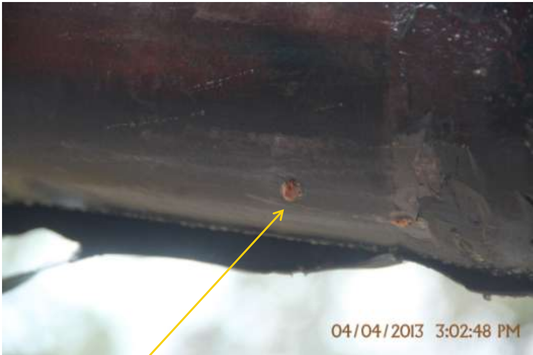
Close up: Leak due to corrosion on Opukushi Well34T flowline at Egbemo-Angalabiri. Picture was taken during Joint Investigation of 4 th April 2013.
