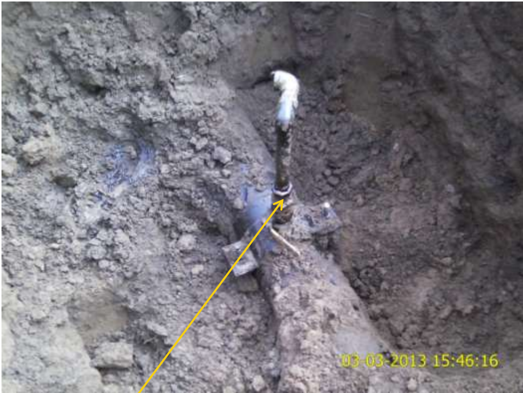
Close up: Illegal fitting on 8" Umuechem – Nkpoku pipeline at Umuwenye. Picture was taken during Joint Investigation of 3 rd March 2013.
