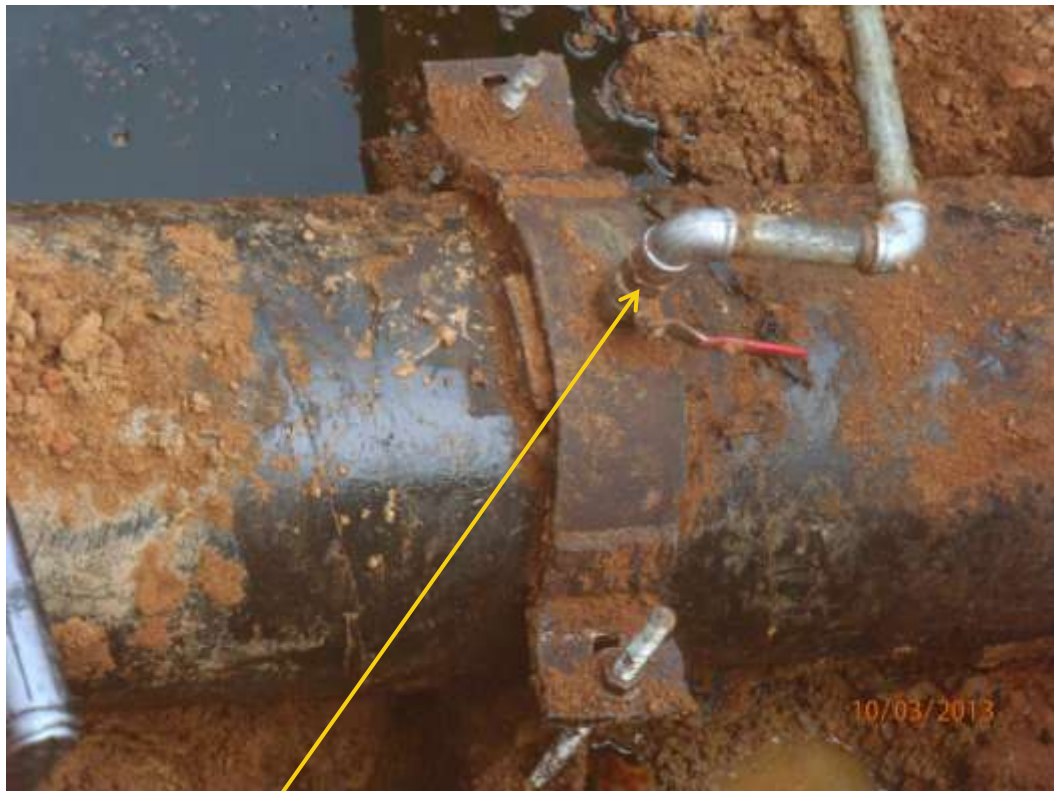
Close up: Illegal fitting on 12" Imo River2 pipeline at Odagwa. Picture was taken during Joint Investigation of 10 th March 2013.
