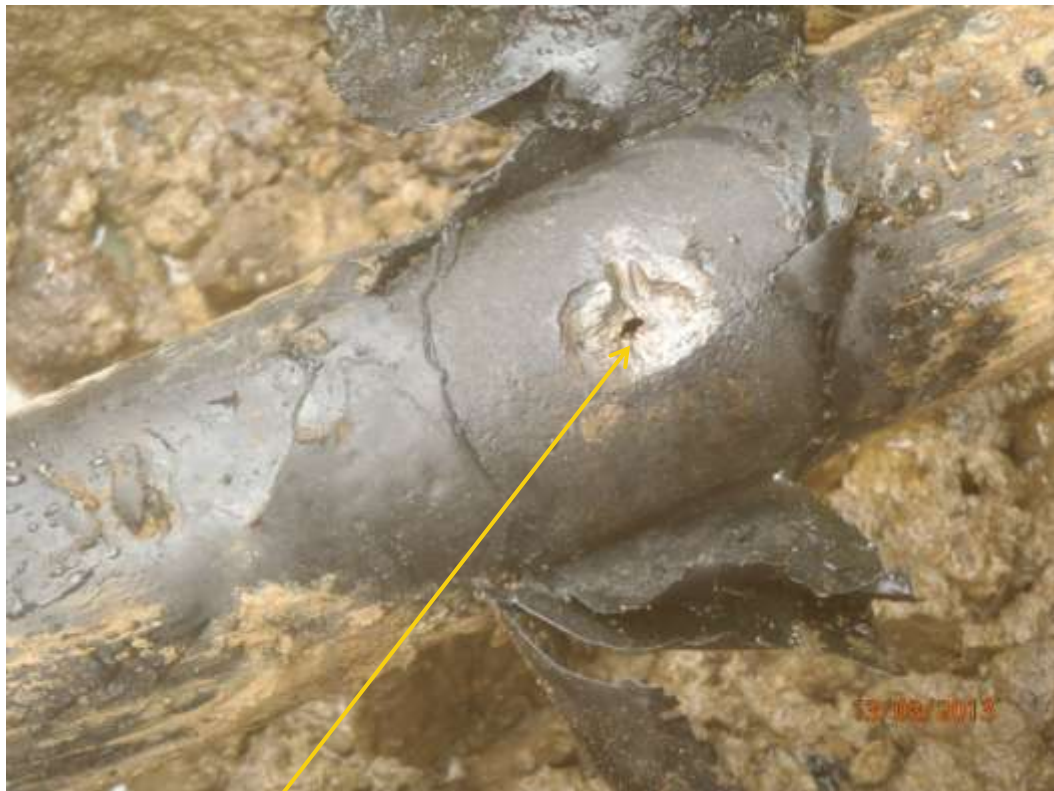
Close up: Drilled hole on Imo River1 Well13L gaslift line at Igirukwu/Isi-Etithoha. Picture was taken during Joint Investigation of 13 th March 2013.
