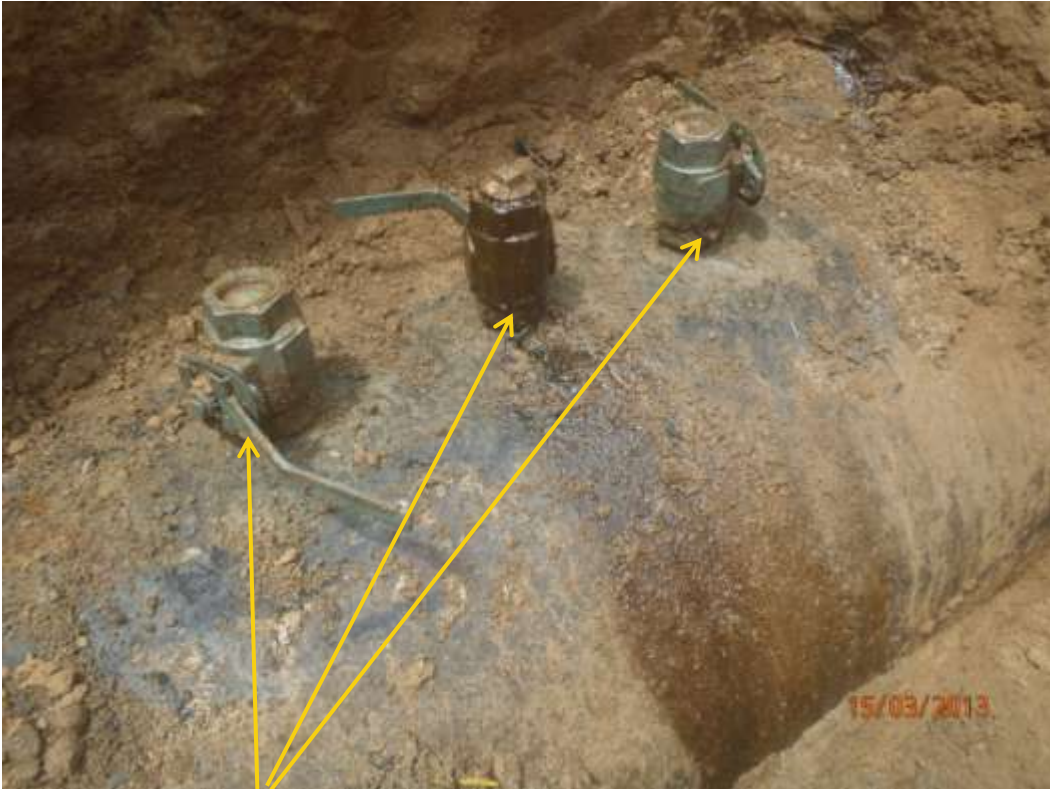
Closeup: Illegal fittings on 36" Nkpoku-Bomu pipeline at Agbonchia. Picture was taken during Joint Investigation of 15 th March 2013.
