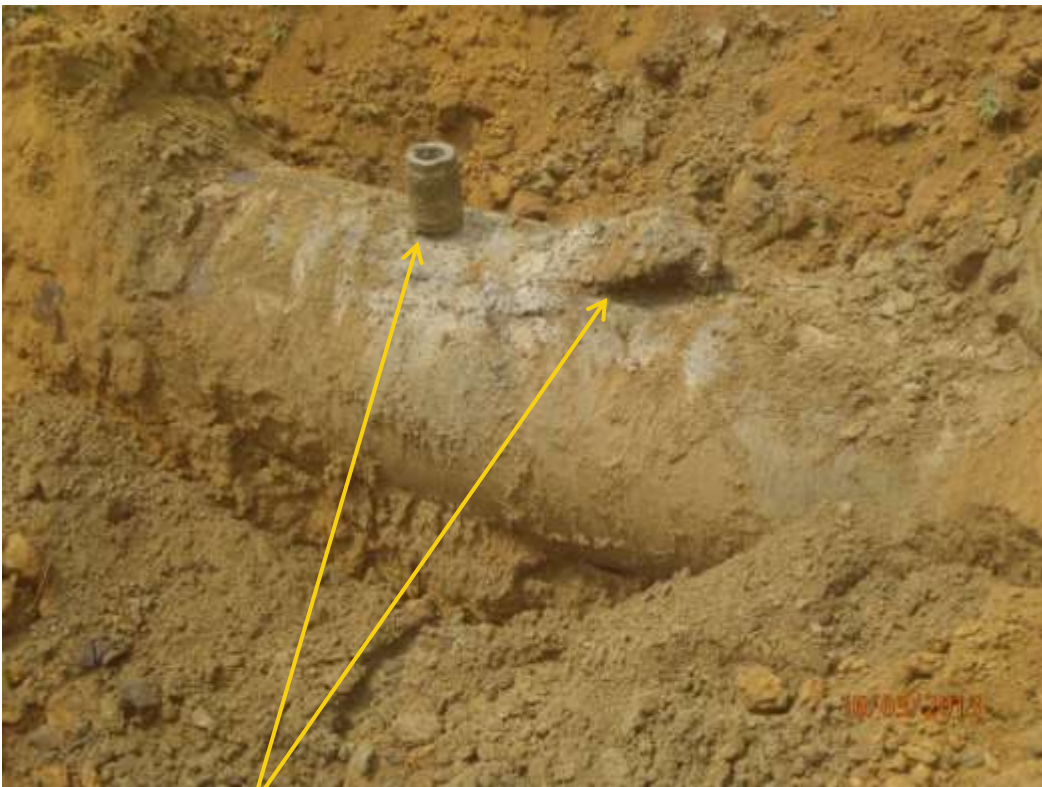
Close up: Illegal fittings on 36" Nkpoku-Bomu pipeline at Agbonchia. Picture was taken during Joint Investigation of 16 th March 2013.
