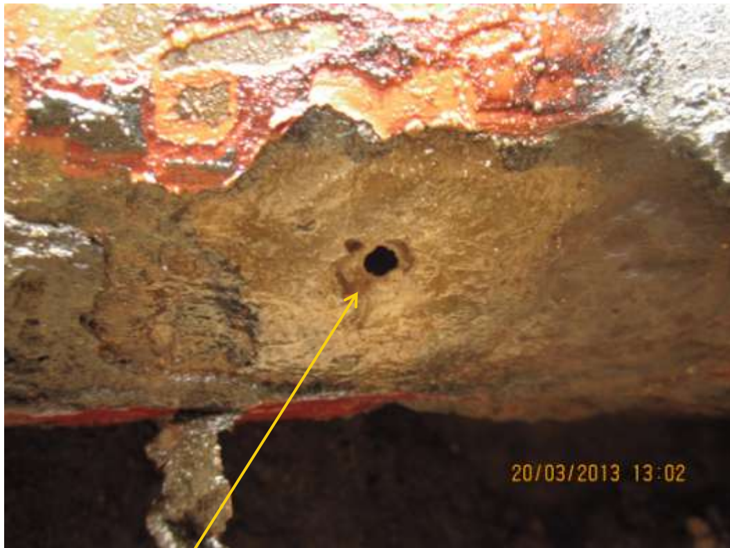
Close up: Leak due to corrosion on Agbada 2 Well66L flowline at Umuokwa. Picture was taken during Joint Investigation of 20 th March 2013.
