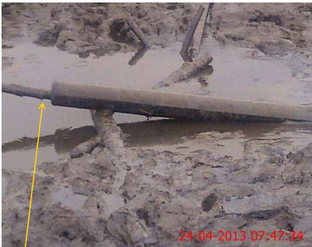
Close up: Missing Flow line on 4" Cawthorne Channel 1 Well 49 Flow line at Mbiama. Picture was taken during Joint Investigation of 24 th April 2013.
