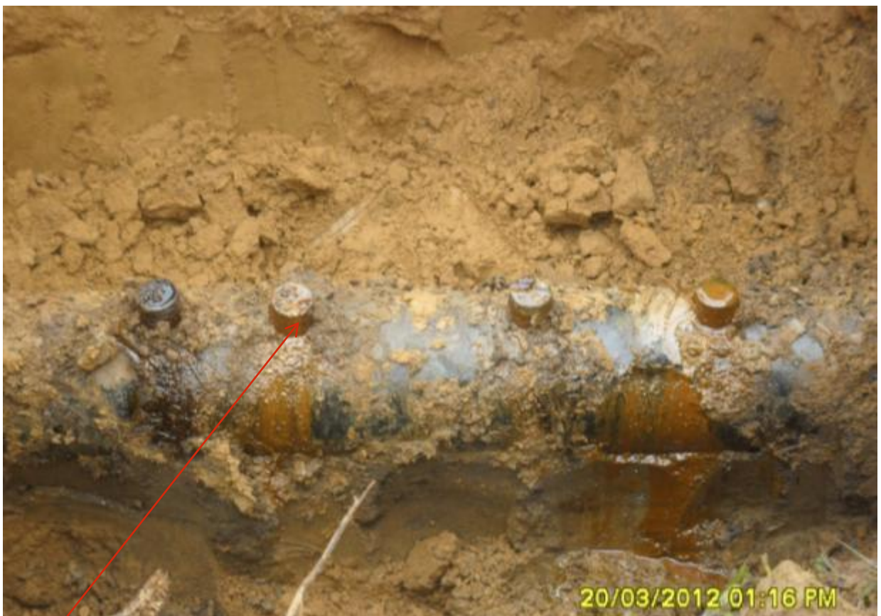
Close-up: Illegal fitting on 8" Isimiri pipeline at Obiakpu. Picture was taken during Joint Investigation of 20 th March, 2012.
