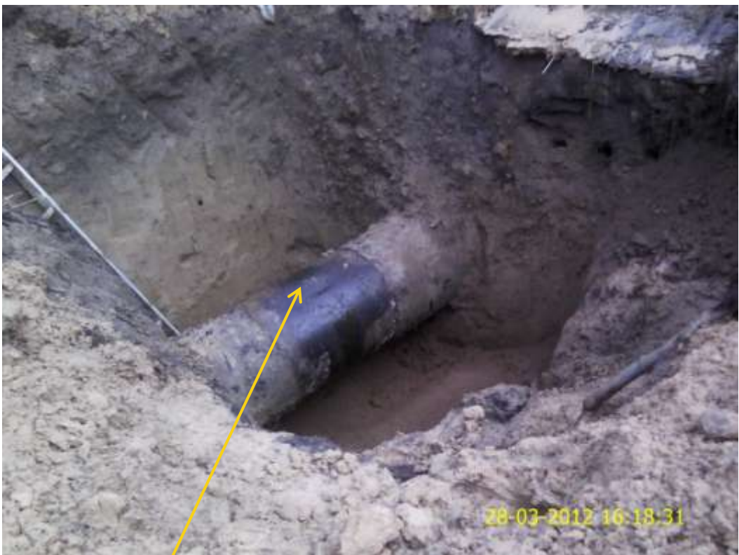
Close up: Hacksaw cut on 24" Bomu-Bonny pipeline at Mogho. Picture was taken during Joint Investigation of 28 th March 2012.
