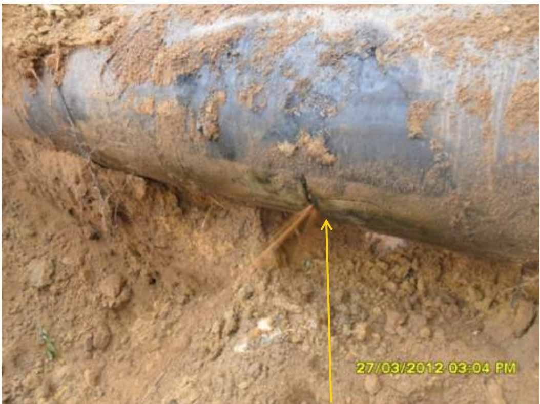
Close up: Hacksaw cut on 24" Nkpoku-Bomu pipeline at Bera. Picture was taken during Joint Investigation of 27 th March 2012.
