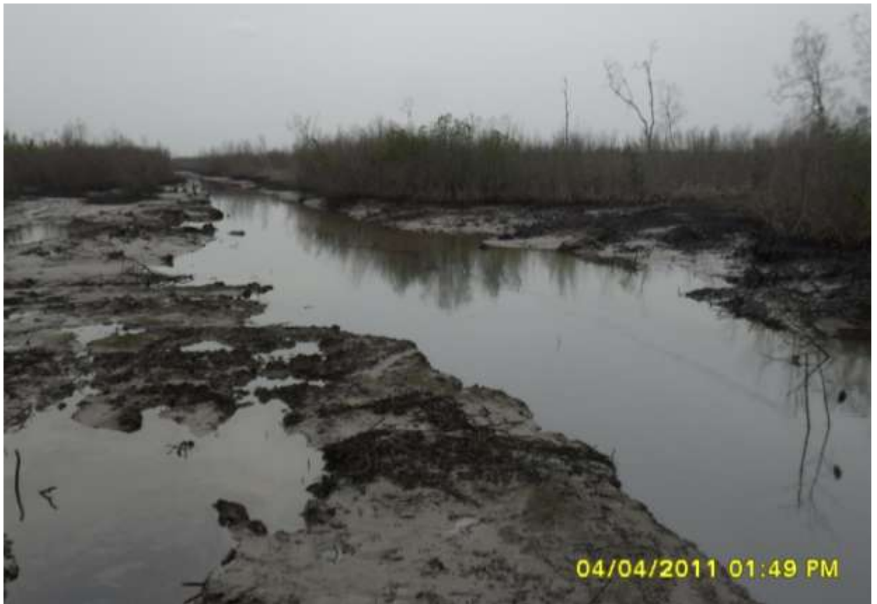
Overview: Extent of the spill incident impact on 24" Alakiri-Bonny Pipeline route at Kalibiama. Pictures taken during Joint Investigation of 4 th - 8 th April, 2011
