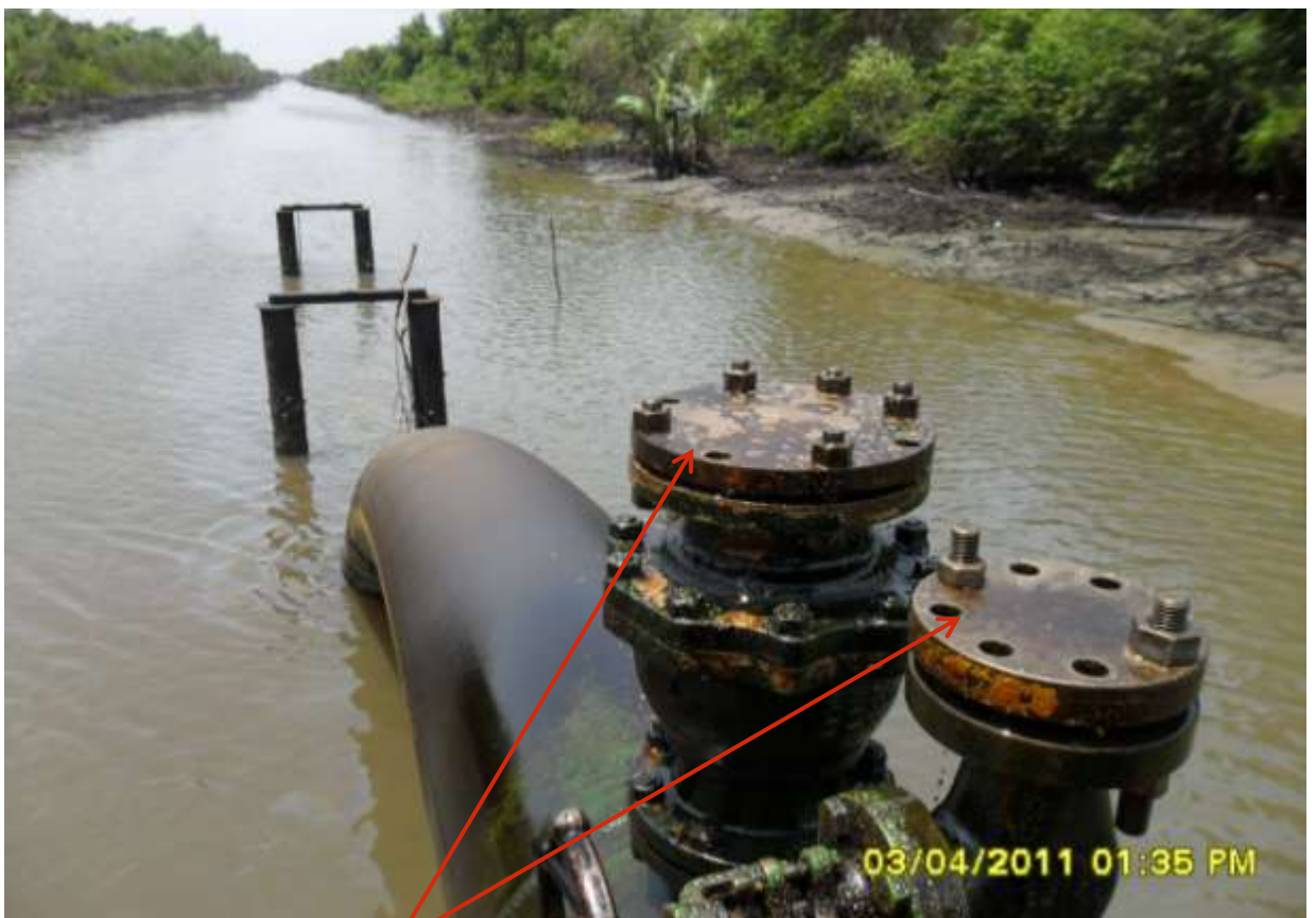
Close-up: Spill due to Tampering with flange nuts & bolts on 24" Cawthorne channel-Bonny Block Valve Station pipeline route at Kalibiama. Pictures taken during Joint Investigation of 1 st - 3 rd April, 2011
