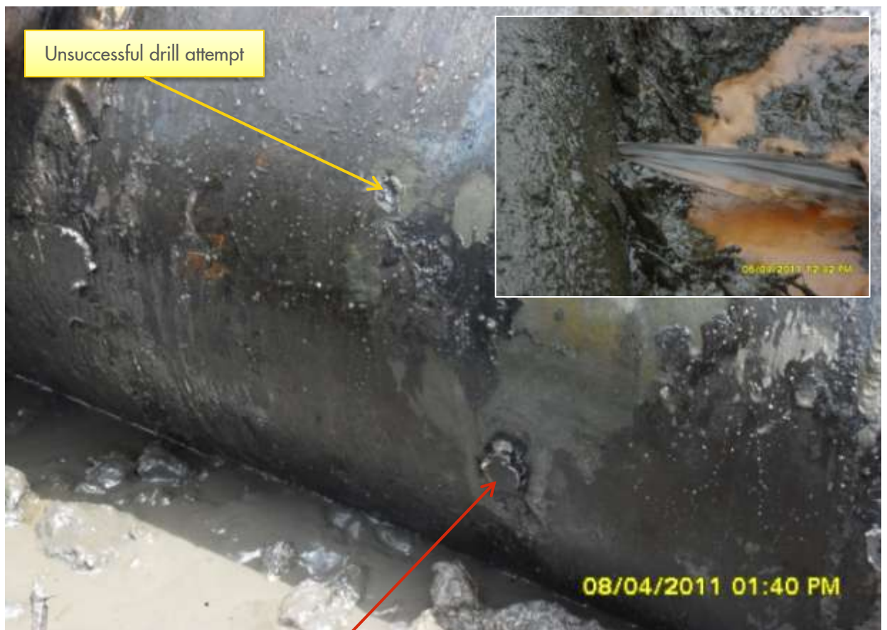
Close-up: Insert shows spill due to drilled hole on 24" Alakiri-Bonny pipeline route at Kalibiama. Main picture shows spill point after plugging. Unsuccessful drill attempt can also be seen.
