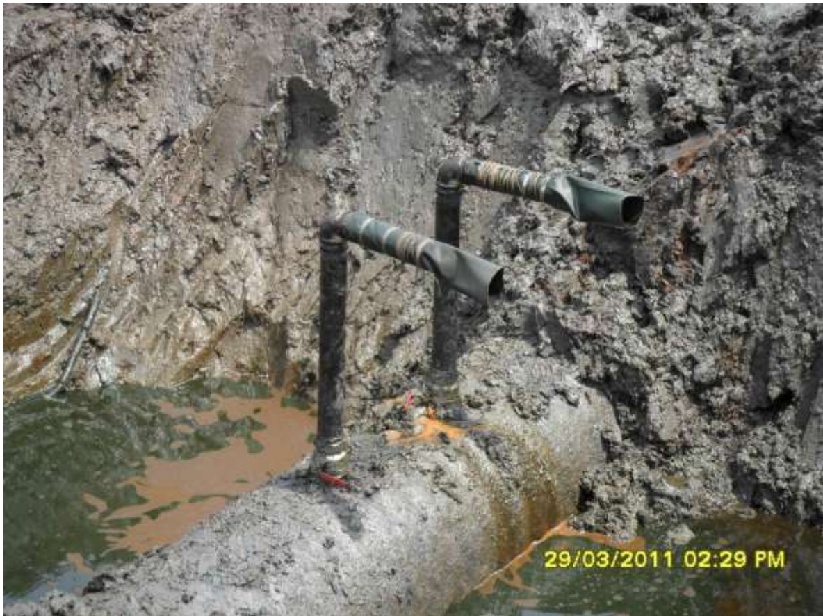
Close-up: Picture showing illegally welded points on 28in Bomu-Bonny pipeline at Bodowest. Picture taken during Joint Investigation of 29 th March, 2011.
