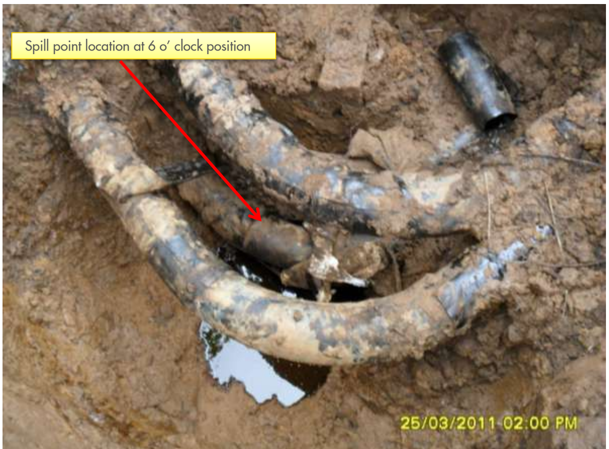
Close-up: Spill due to corrosion on Umuechem well 22T Flowline at Umuechem. Picture taken during Joint Investigation of 25 th March, 2011.
