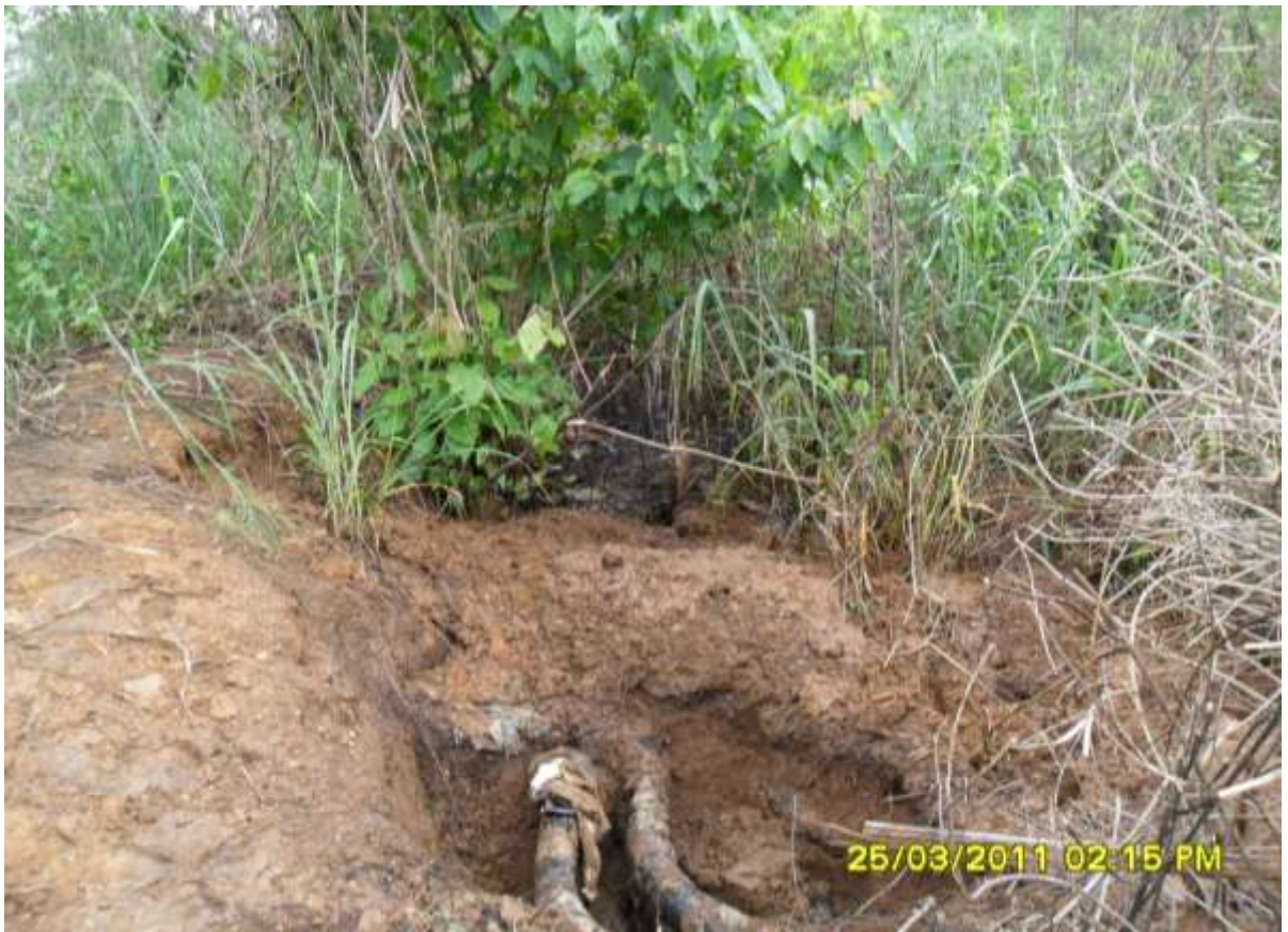
Overview: Extent of the spill incident impact on Umuechem well 22T Flowline route at Umuechem. Picture taken during Joint Investigation of 25 th March, 2011
