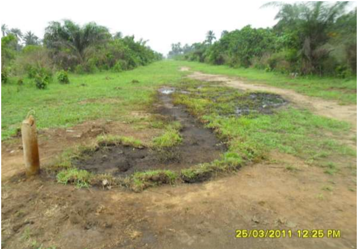
Overview: Extent of the spill incident impact on 8" Obigbo-North Pipeline at Obigbo . Pictures taken during Joint Investigation of 25 th March, 2011
