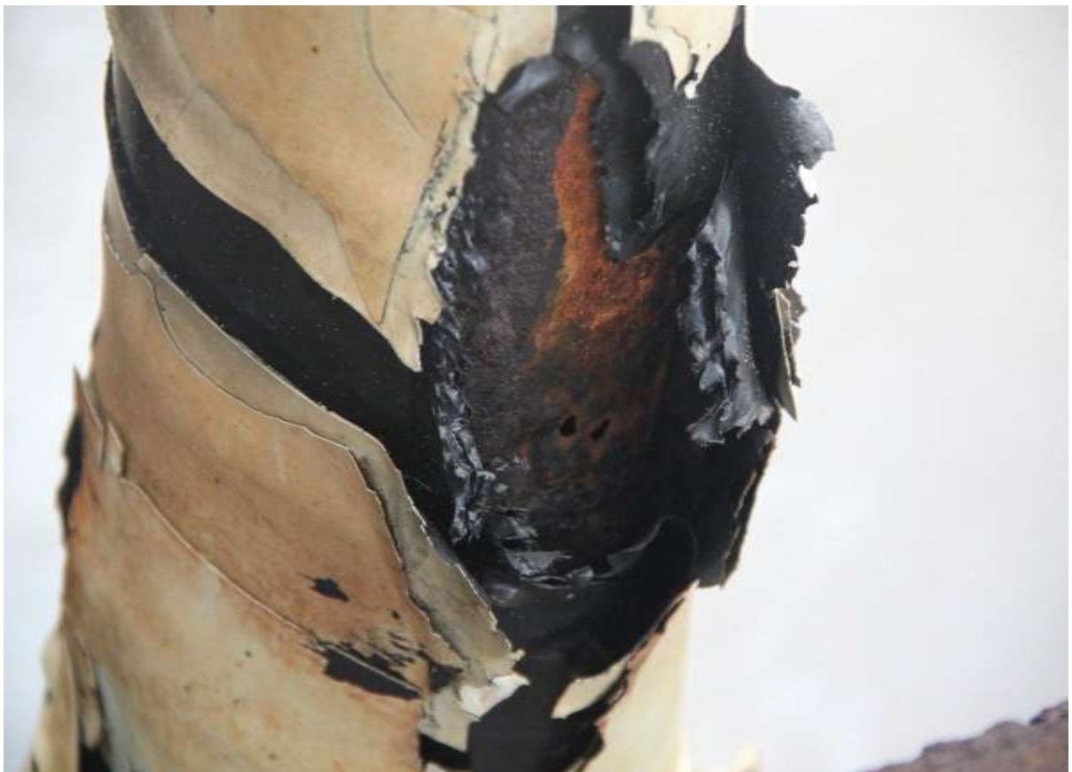
Close-up: Spill due to corrosion on Otumara W-44S Wellhead riser .Picture taken during Joint Investigation of 28 th March, 2011.
