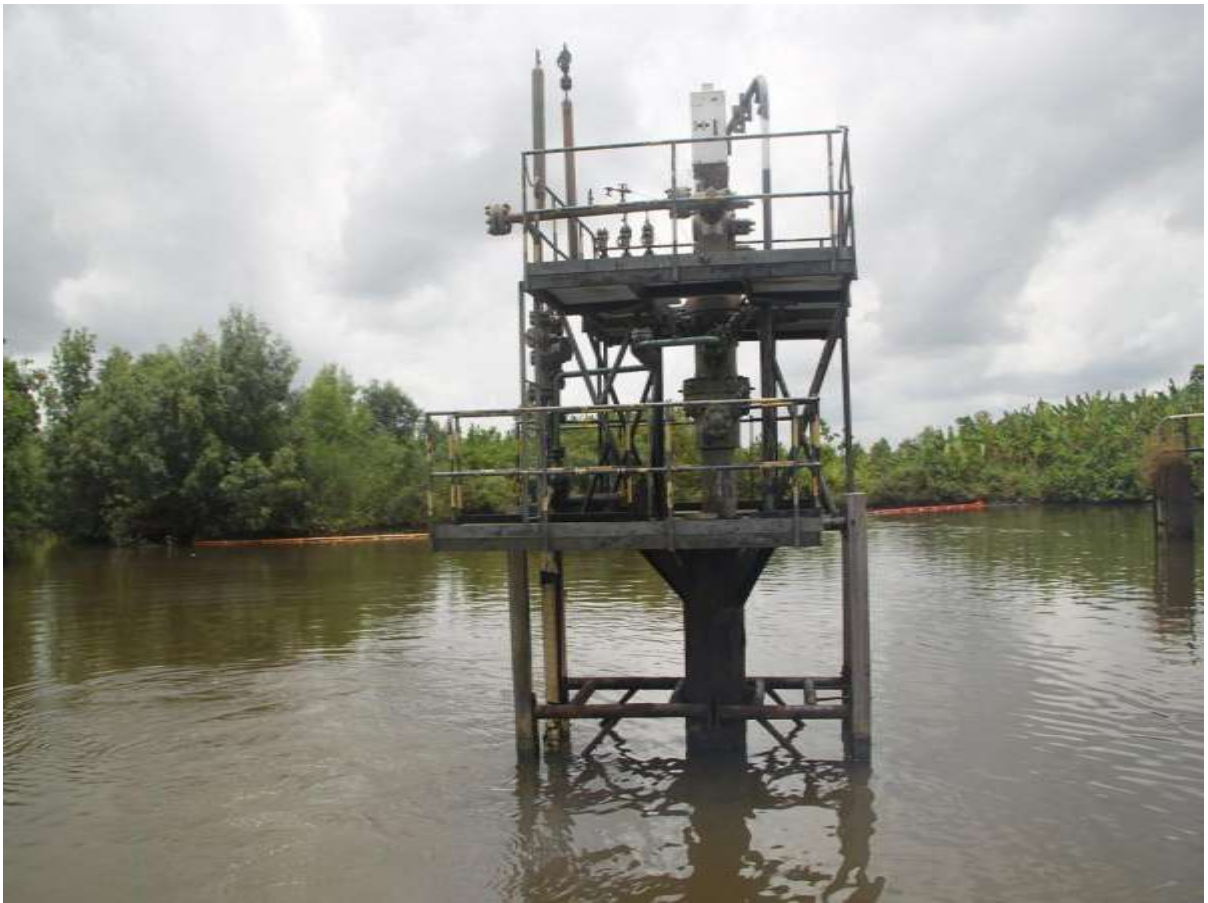
Overview: Extent of the spill incident impact on Otumara W-44S Wellhead riser. Pictures taken during Joint Investigation of 28 th March, 2011
