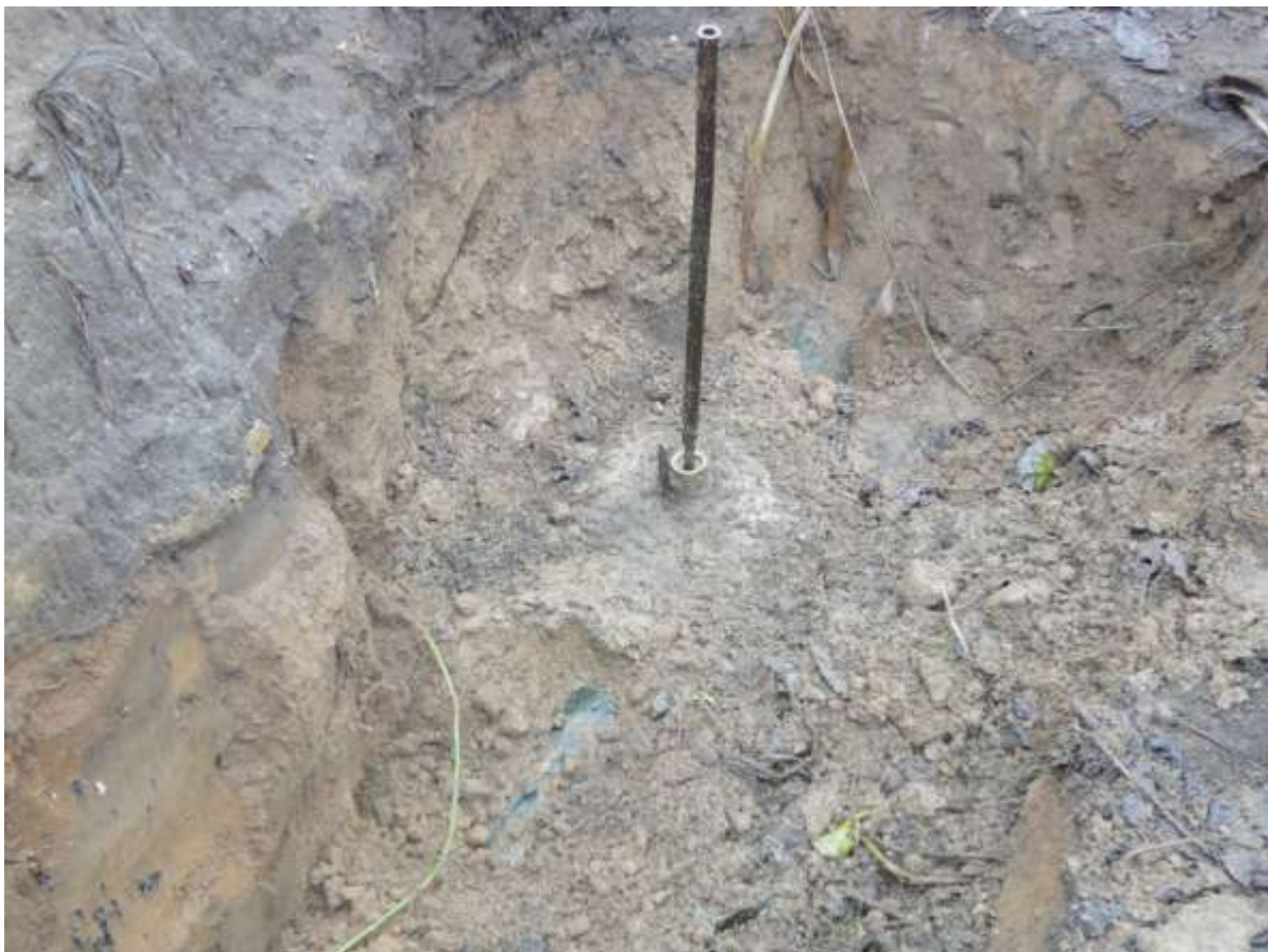
Close-up: Illegally welded point on Imo River 1 Well 59T Flowline. Picture was taken during JIV of 15 March 2011
