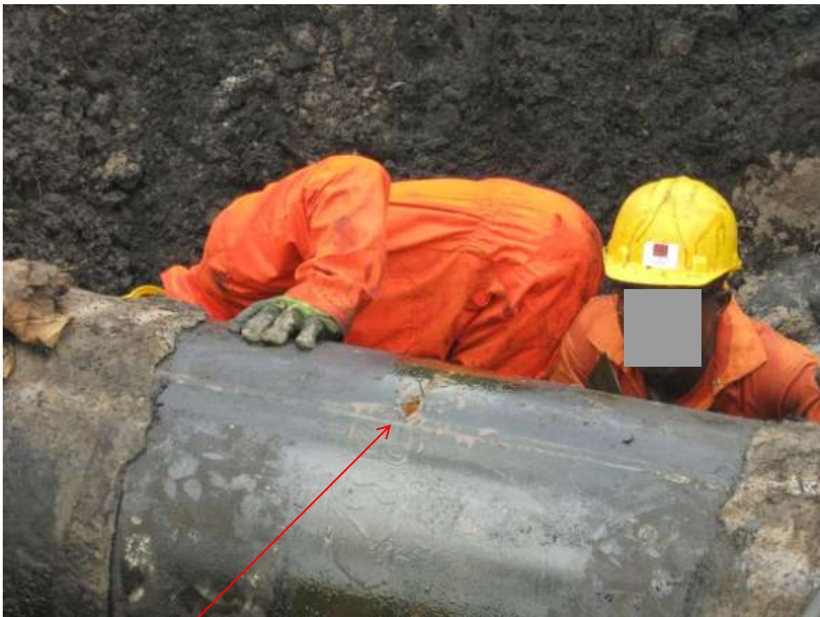
Close-up: Hacksaw cut on 24' Bomu-Bonny Pipeline at K-Dere. Picture was taken during JIV of 11 March 2011
