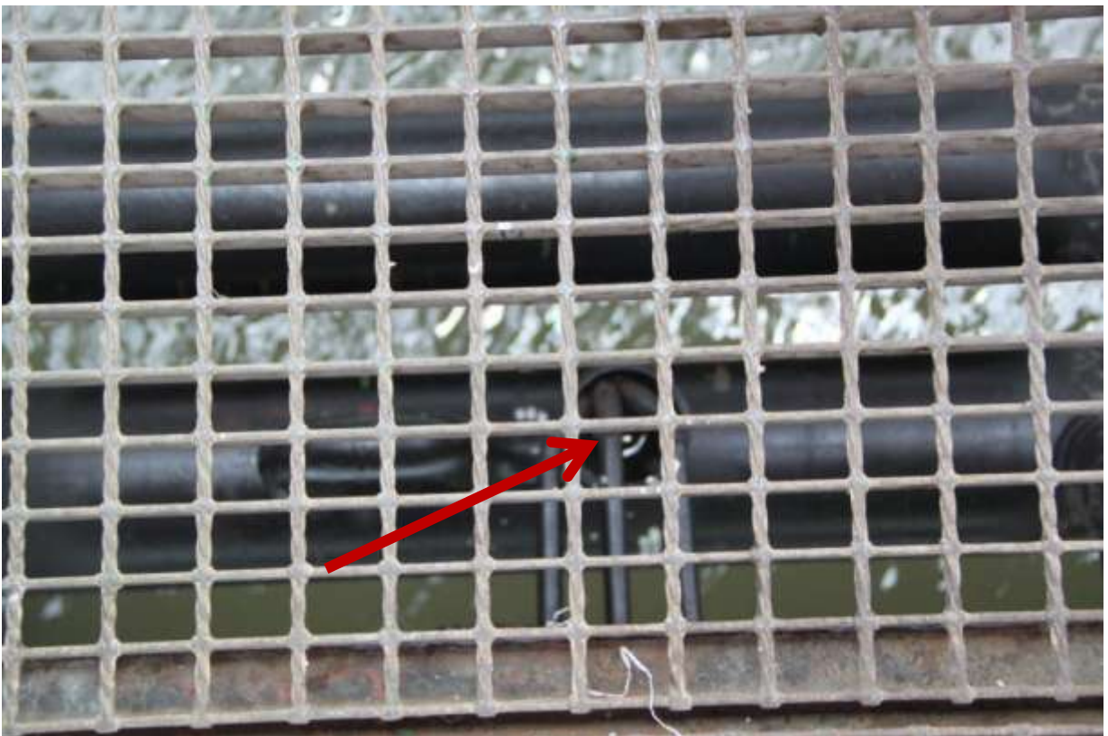
Close-up: Showing spill point at Batan Flowstation spill in Batan. Picture was taken during JIV of 11 March 2011
