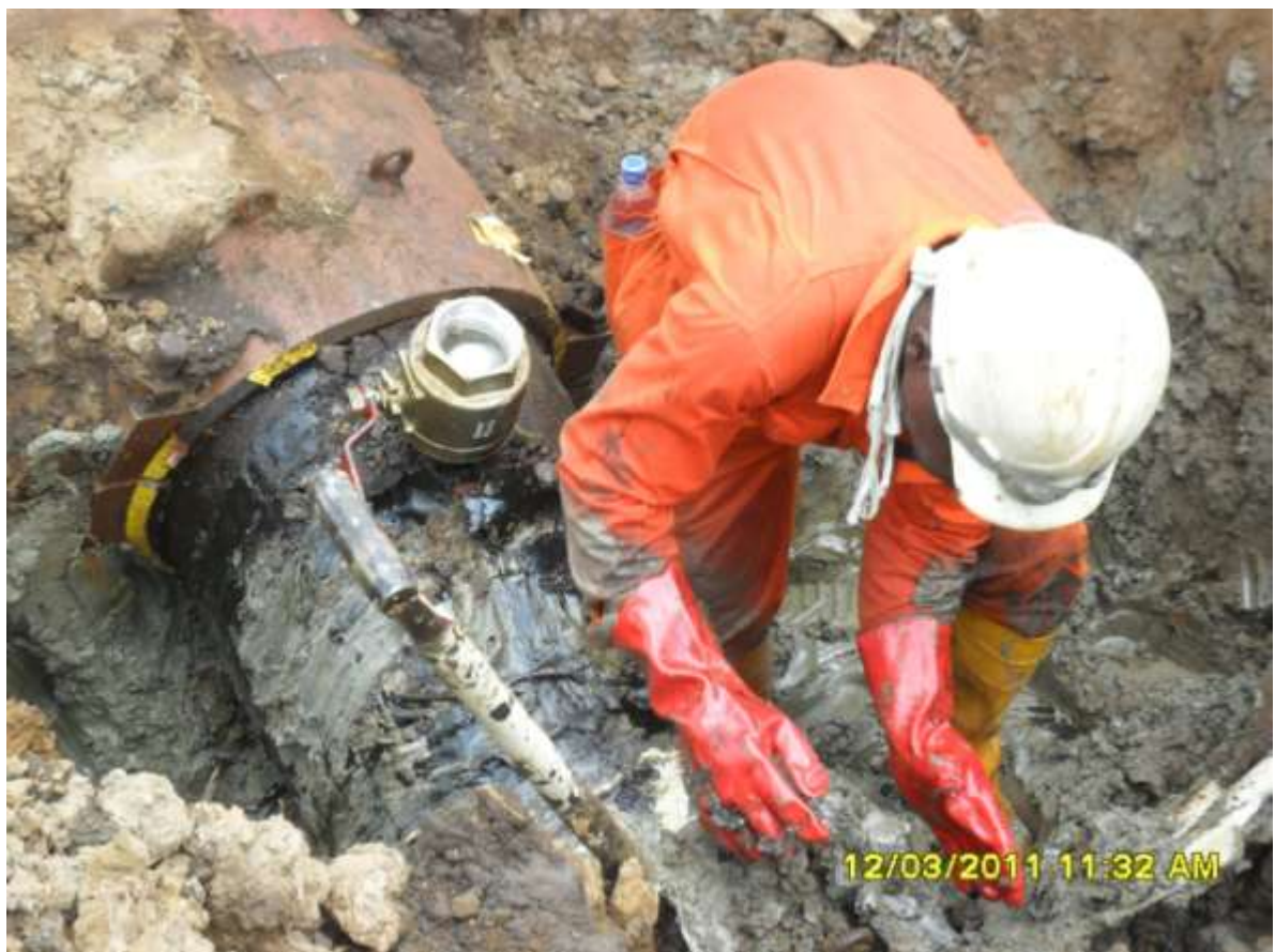
Close-up: Illegally welded point on 20' Kolocreek-Rumuekpe Pipeline at Ogbogolo. Picture was taken during JIV of 12 March 2011
