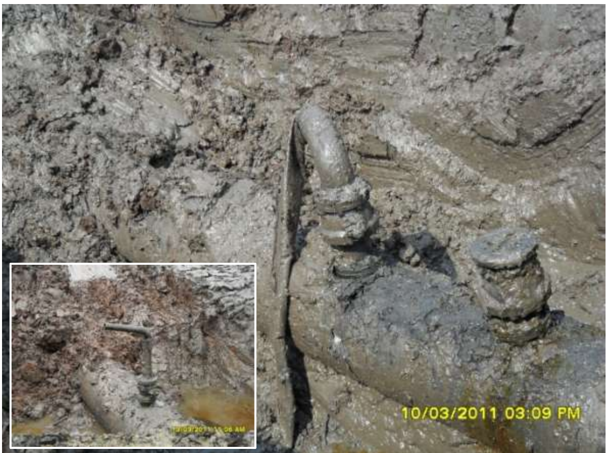
Close-up: Illegally welded points on 24' Bomu-Bonny Pipeline at Bodo West. Insert showing illegally welded points on 28' Bomu-Bonny Pipeline at Bodo West. Pictures taken during JIV of 10 March 2011.
