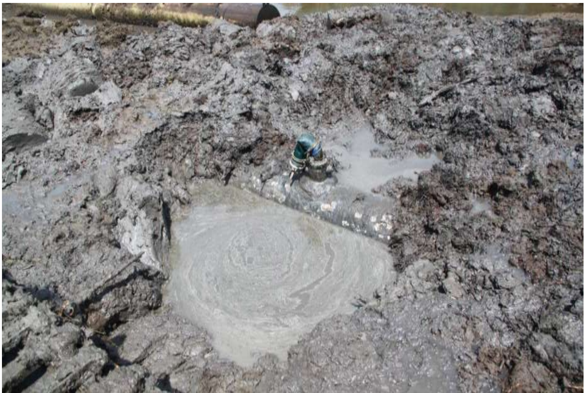
Close-up: Illegally welded point on 28" Trans Forcados Pipeline route in Chanomi. Picture was taken during JIV of 10 March 2011
