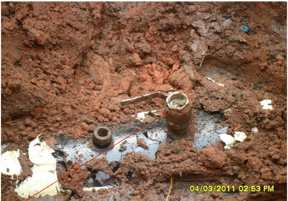
Close-up: Spill due to illegally welded points on 16" Egbema-Assa Pipeline at Assa. Picture taken during Joint Investigation of 4 th March, 2011 .
