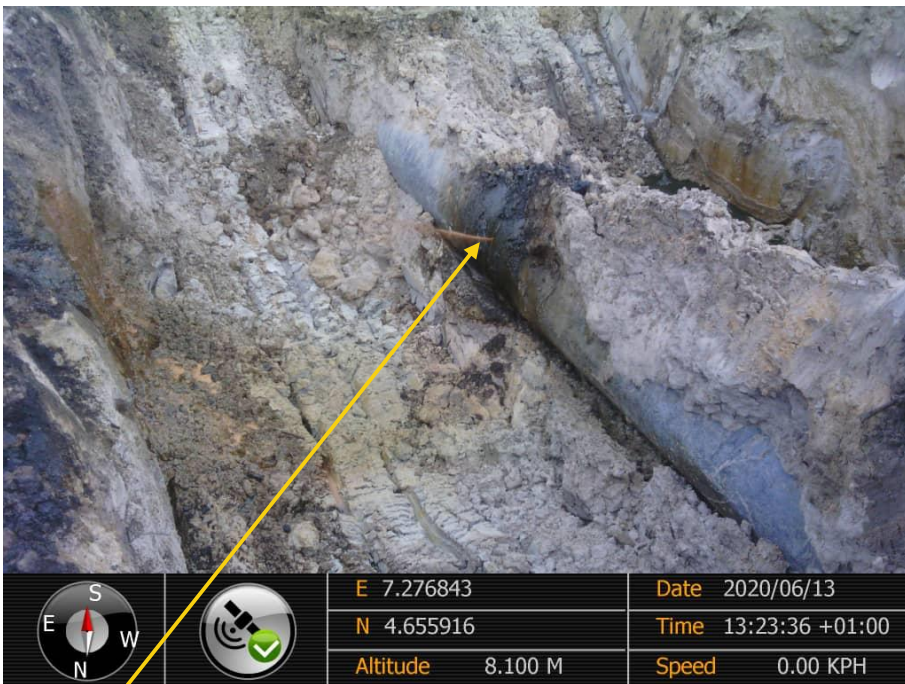
Close-up: Hack saw cut of 4m at 3 o'clock position on 28" Bomu Bonny Pipeline at Kpor. Picture was taken during Joint Investigation of 13 th June 2020.
