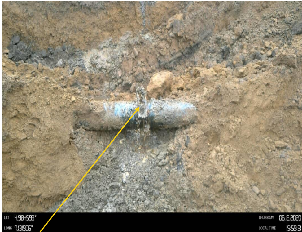
Close-up: 1.5" bulb valve installed at 12 o'clock position on 8" Nkali - ImoRiver Deliveryline at Odagwa. Picture was taken during Joint Investigation 18th June 2020.
