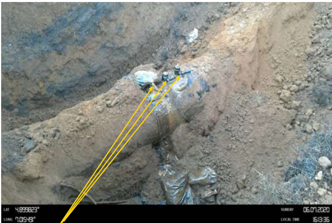
Close-up: 3 nos 2" valves installed at 12 o'clock position on 28" Nkpoku Bomu Pipeline at Rumuowha. Picture was taken during Joint Investigation 7th June 2020.
