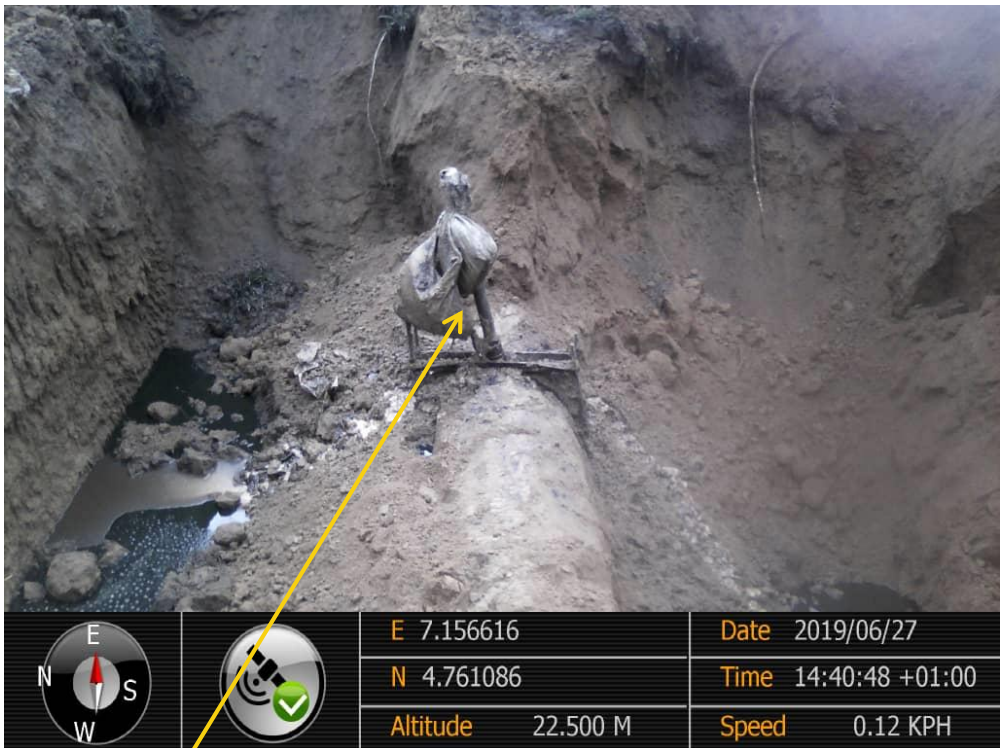
Close-up: Illegal fitting on 28'' Nkpoku - Bomu Pipeline at Ejamah – Ebubu. Picture was taken during Joint Investigation of 27 th June 2019.
