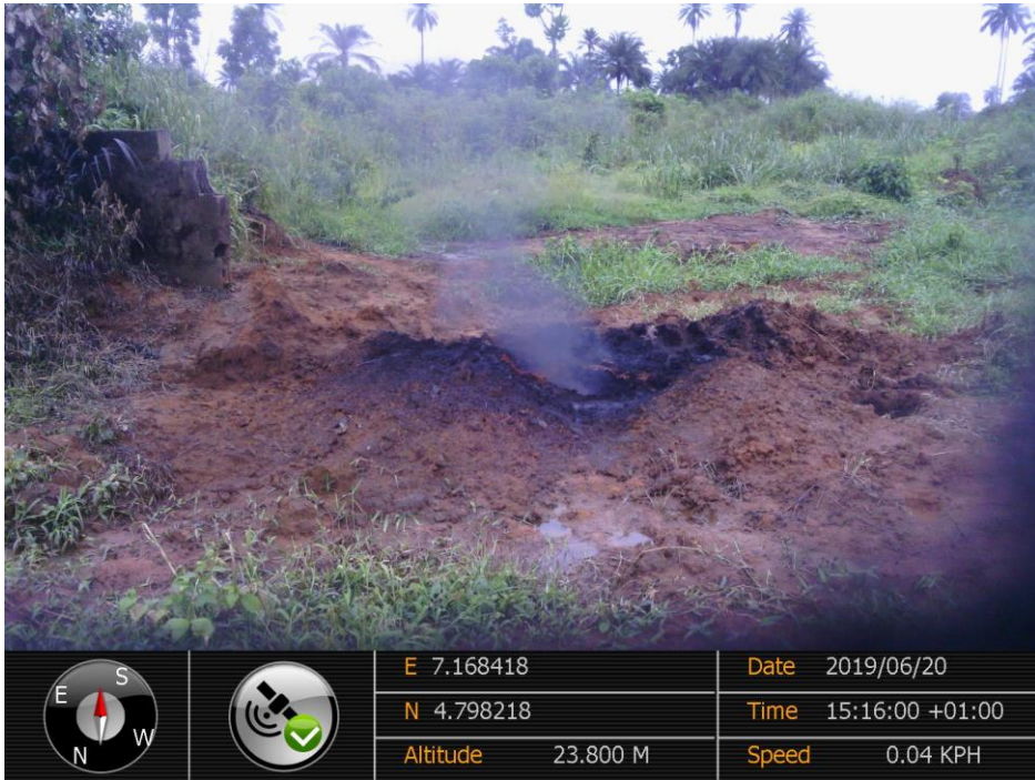
Overview: Part of spill impact on 24" Nkpoku-Bomu Pipeline Right of Way at Egbalor. Picture was taken during Joint Investigation of 20 th June 2018.
