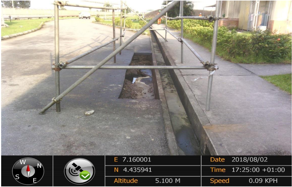
Overview: Part of spill impact on 16" Bonny Disused Export Pipelines at Bonny. Picture was taken during Joint Investigation of 2 nd August 2018.
