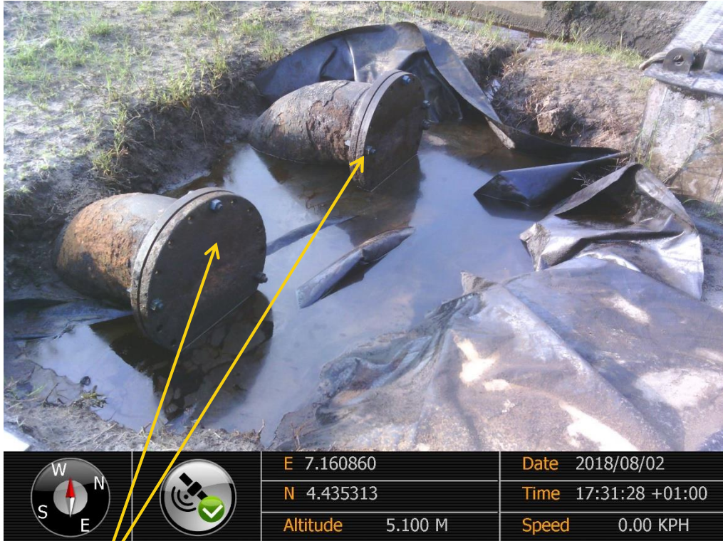
Close-up: Corroded Disused 16" Flanges on 16" Bonny Disused Export Pipelines at Bonny. Picture was taken during Joint Investigation of 2 nd August 2018.
