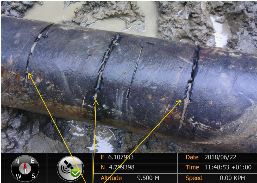
Close-up: Leaking multiple Hacksaw Cuts on 10'' DiebuCreek– Nun River Pipeline at Oporoma. Picture was taken during Joint Investigation of 22 nd June 2018.
