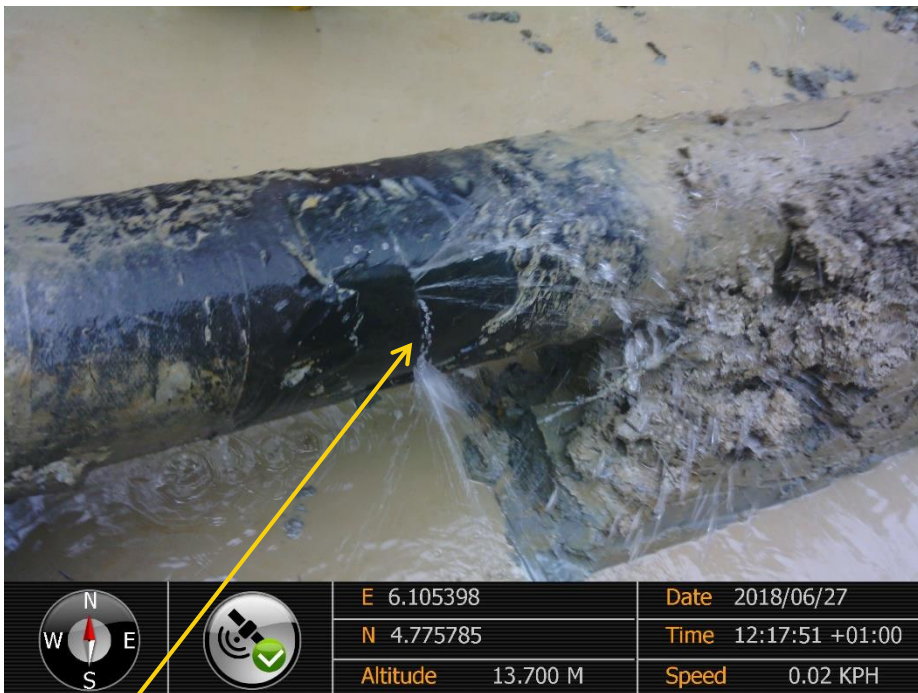
Close-up: Hacksaw Cut on 10'' DiebuCreek– Nun River Pipeline at Oporoma. . Picture was taken during Joint Investigation of 27 th June 2018.
