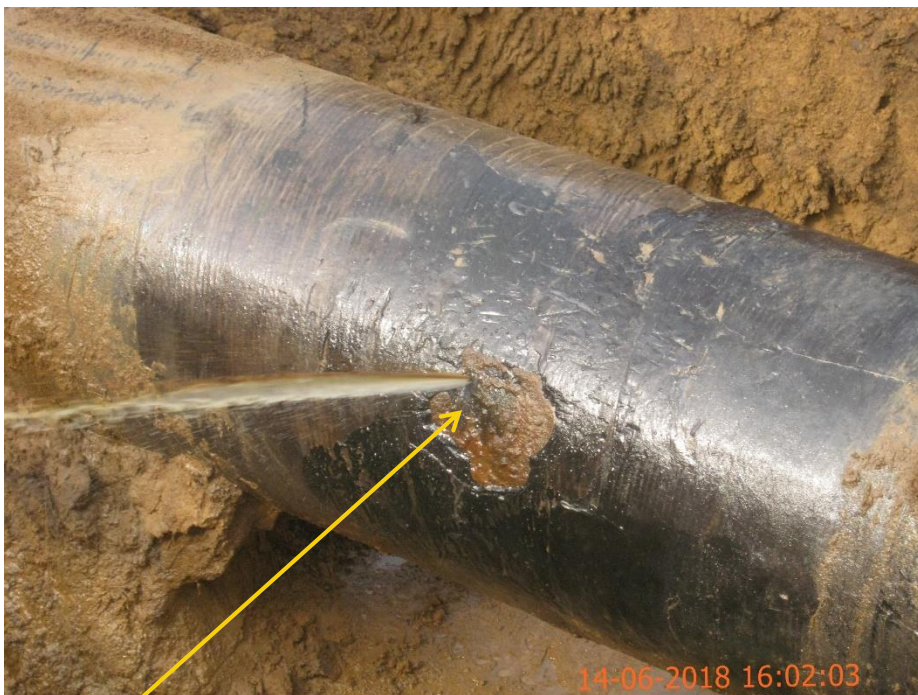
Close-up: Drilled Hole on 24" Nkpoku-Bomu Pipeline at B-Dere. Picture was taken during Joint Investigation of 14 th June 2018.
