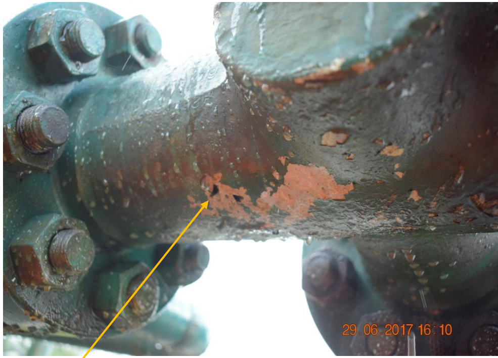
Close-up: Corrosion on Tunu Well 7T Wellhead at Agbidiama. Picture was taken during Joint Investigation of 29 th June 2017.
