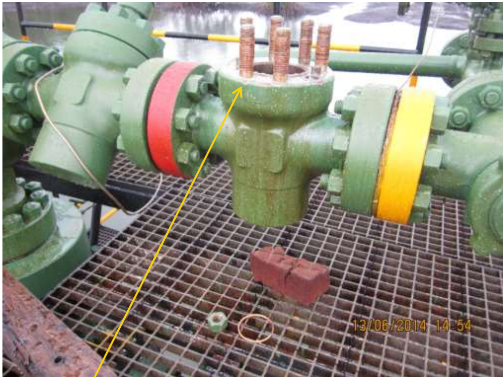
Close-up: Original position of control unit removed from Belema Well9T Wellhead at Belema. Picture was taken during Joint Investigation of 13 th June 2014.
