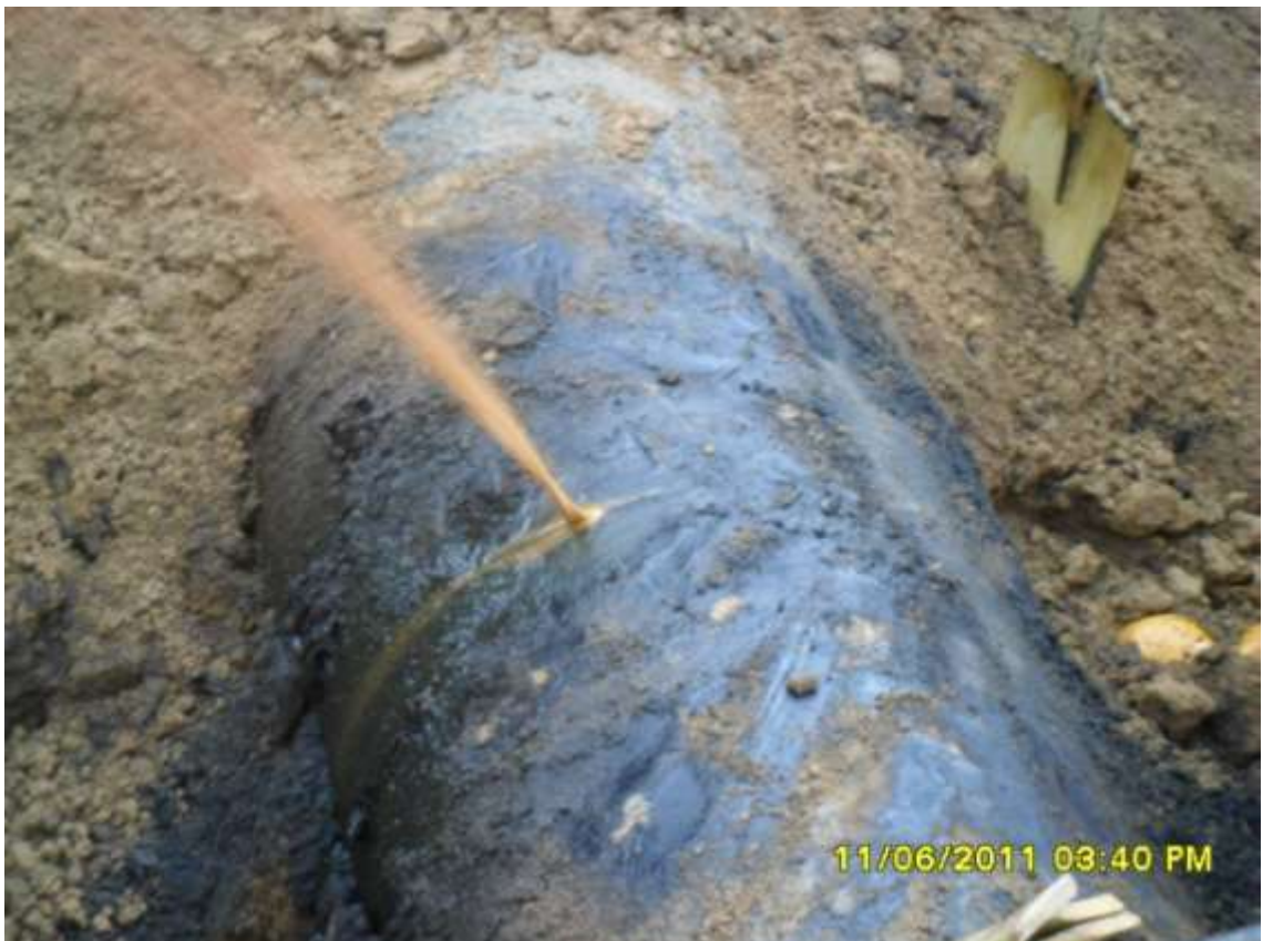
Close-up: Leak point on 28 inch Bomu-Bonny Trans Niger pipeline at Mogho. Picture taken during Joint Investigation of 11 th June, 2011.
