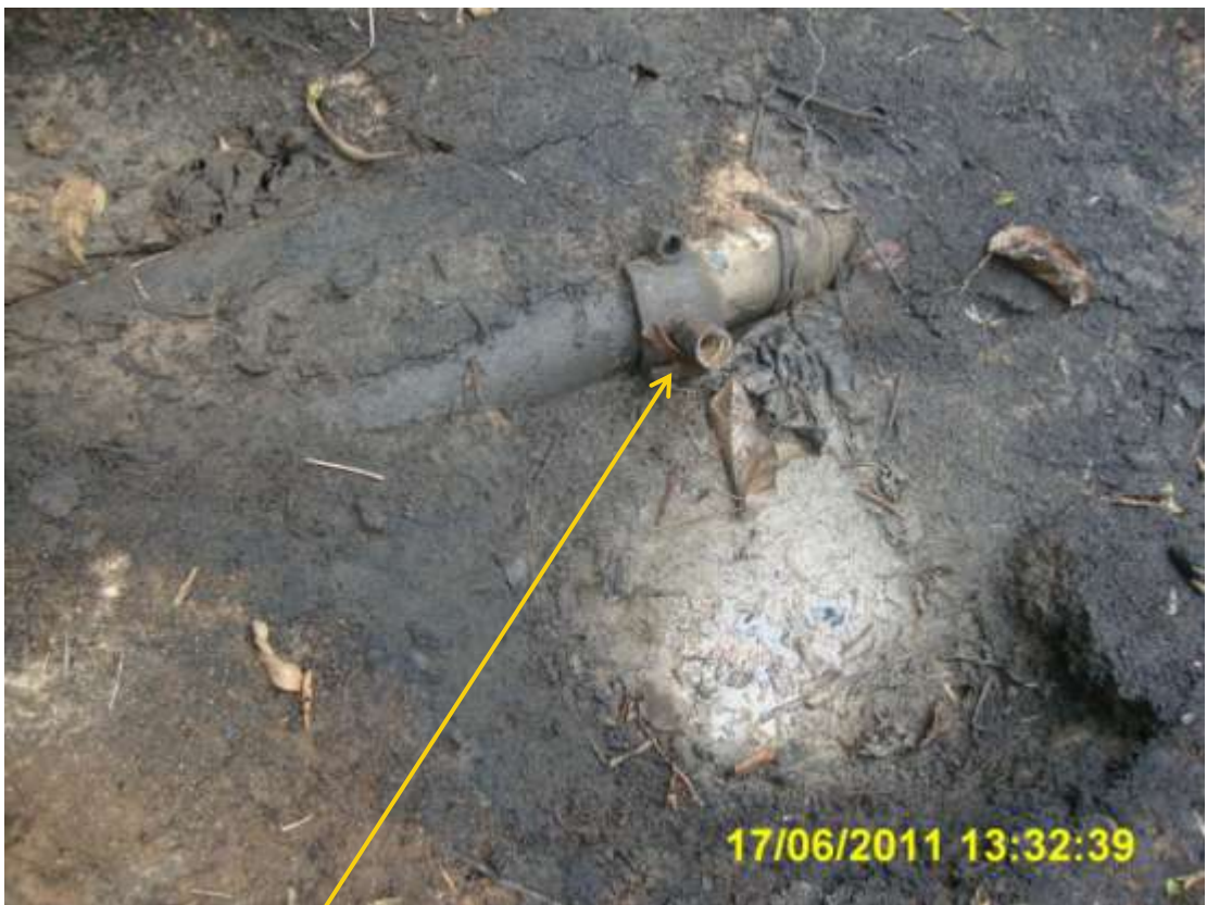
Close-up: Illegally welded fitting on Well56L flowline at Isietitioha. Picture taken during Joint Investigation of 17 th June, 2011
