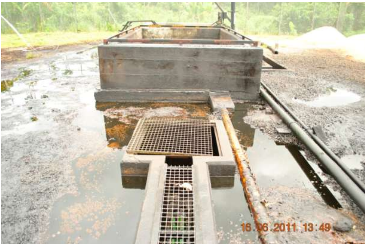
Close-up: Closeup of sump pit chamber and sump pit at Olomoro compressor station 2 at Olomoro. Picture taken during Joint Investigation of 16 th June, 2011
