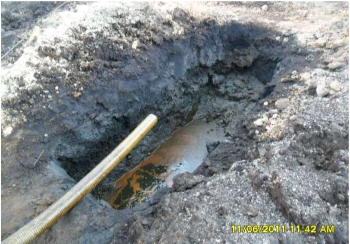
Overview: Part of extent of the spill incident impact on 28'' Bomu-Bonny Pipeline at Bodo (Ogoni) . Picture taken during Joint Investigation of 11 th June, 2011
