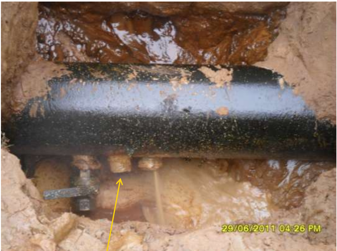
Close-up: Spill due to illegal fittings on 12" Imoriver pipeline at Uzuaku. Picture taken during Joint Investigation of 29 th June, 2011
