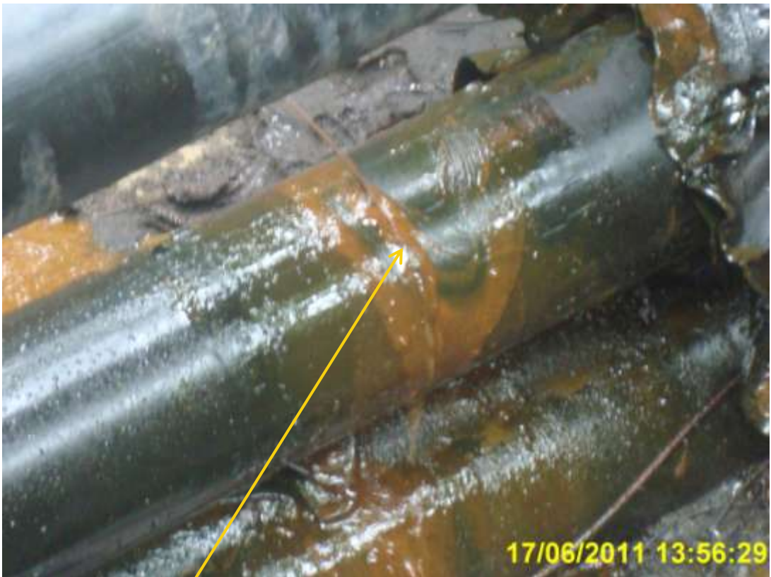
Close-up: Hacksaw cut on Imo River Well 55S flowline at Igiriukwu. Picture taken during Joint Investigation of 17 th June, 2011
