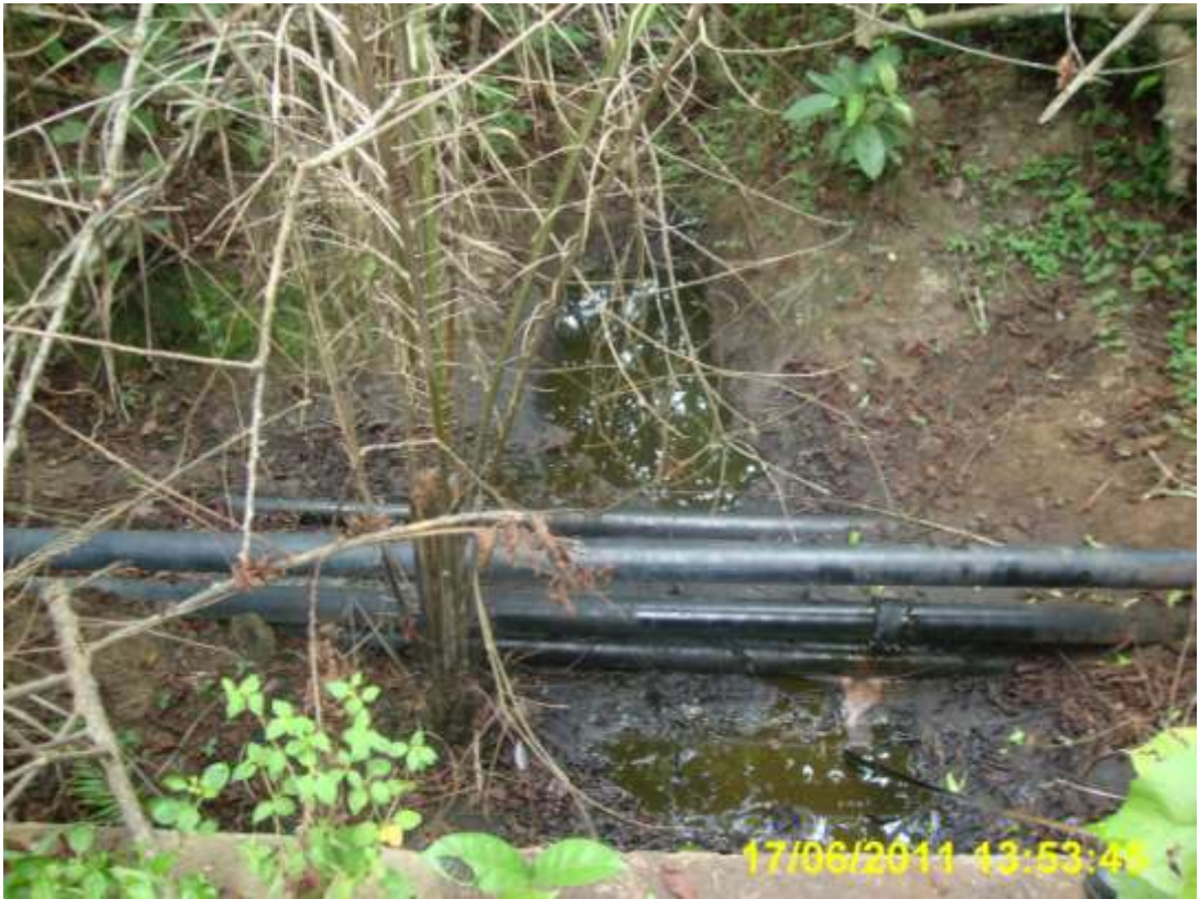
Overview: Part of the spill impact on Imo River Well 55S flowline at Igiriukwu. Picture taken during Joint Investigation of 17 th June, 2011
