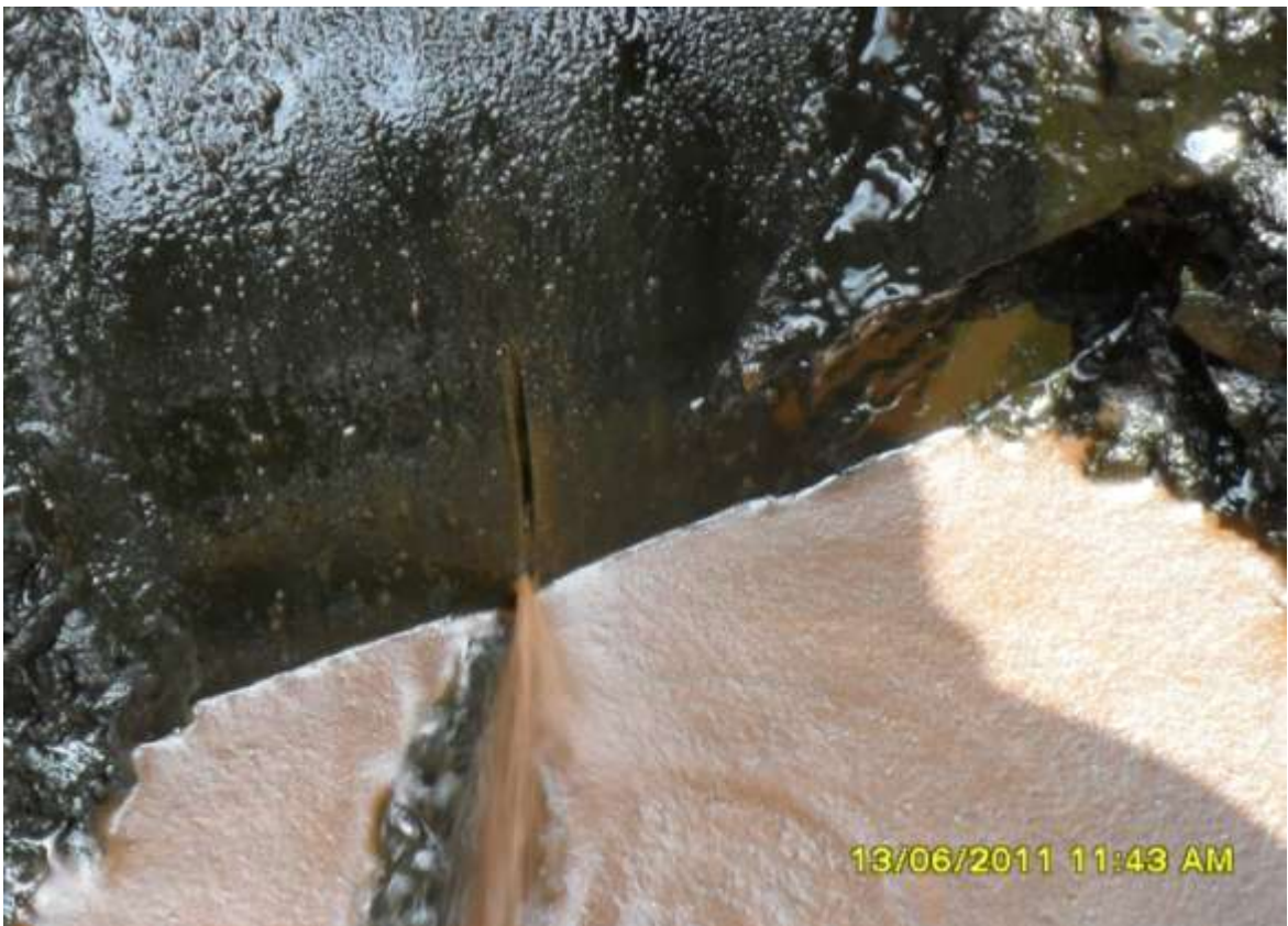
Close-up: Spill due to cut on 24" Bomu-Nkpoku Pipeline at Bera (Ogoni). Picture taken during Joint Investigation of 13 th June, 2011.
