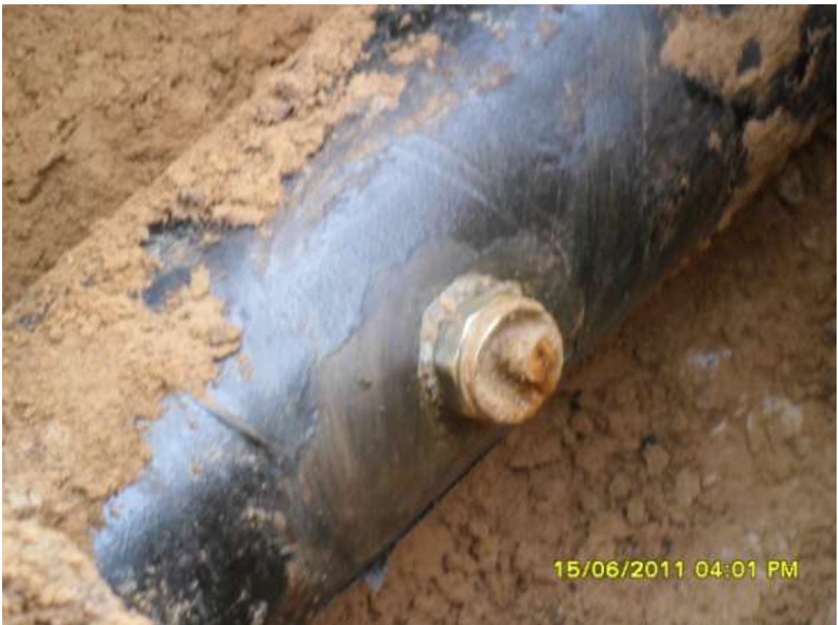
Close-up: Spill due to illegally welded nipple at 2 o'clock position on 12" Imo River1 to Oghale pipeline at Owaza. Picture taken during Joint Investigation of 15 th June, 2011
