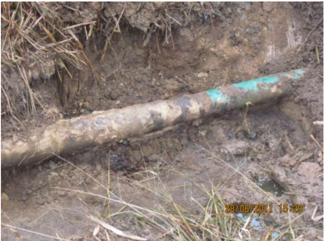
Close-up: Spill due to corrosion on Obigbo Well20T flowline at Umuebule. Picture taken during Joint Investigation of 28 th June, 2011
