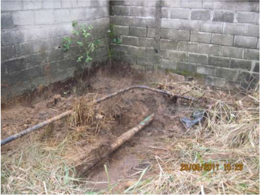
Overview: Impacted area within Obigbo Well20T wellhead facility at Umuebule. Picture taken during Joint Investigation of 28 th June, 2011
