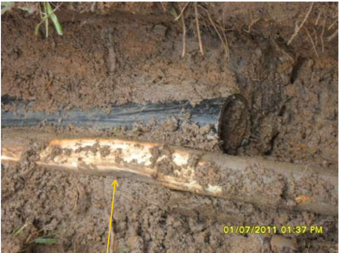
Close-up: Spill due to cut pipe on Imoriver2 Well28L flowline at Umuedeokware. Picture taken during Joint Investigation of 1 st July, 2011
