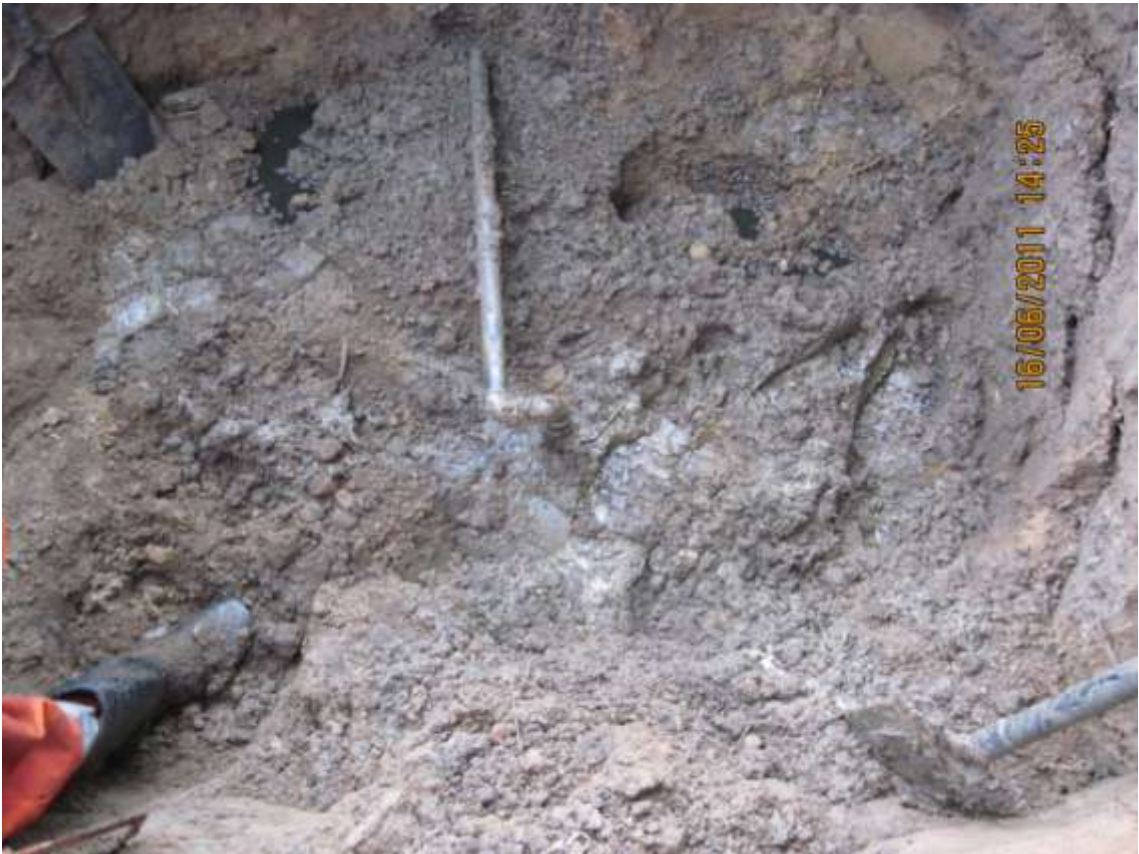
Close-up: Illegally welded fitting at 12 o'clock position on 12" ImoRiver2 pipeline at Owaza. Picture taken during Joint Investigation of 16 th June, 2011
